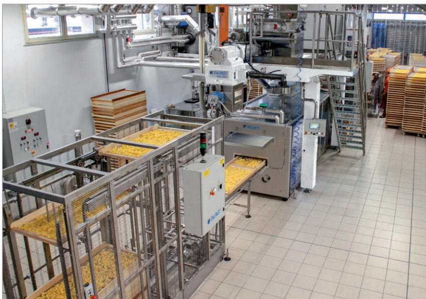
Production line for Pasta, equipped with SOGEVAC FP pumps. With courtesy of company ITALPAST S.r.l., Parma, Italy.
